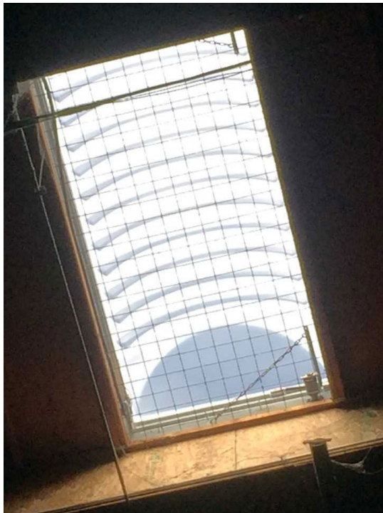
Exhibit 7: Skylight with screen, installed after the fatality.
