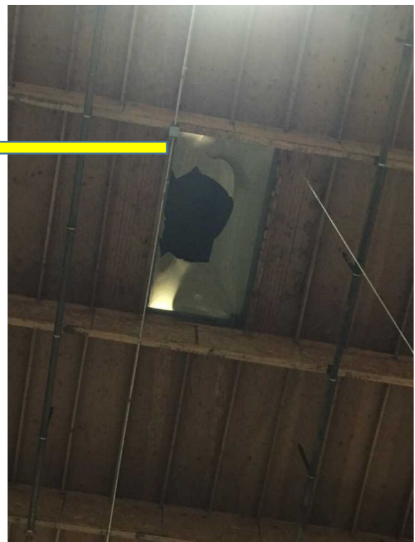
Exhibit 6. Close-up of broken skylight from inside the warehouse.
