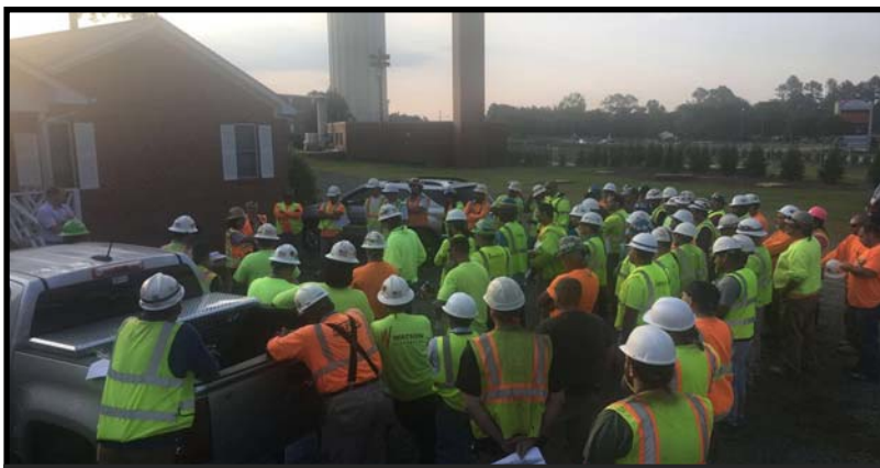
Ann Johnson leads a fall prevention stand-down at a TA Loving wastewater treatment plant project in Columbia, South Carolina
