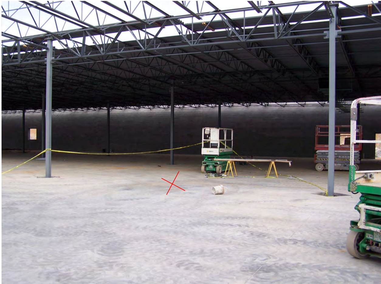
Location where foreman fell.
