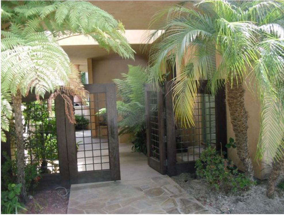
Exhibit 3. The breezeway entry where the victim fell through the opening in the roof.
