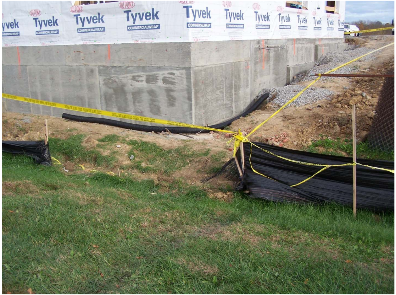
Area of impact where employees landed from fall. Photograph property of KY FACE Program
