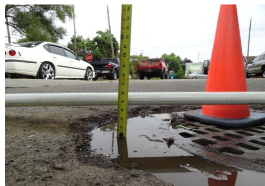
Figure 4. Storm drain cover/pavement condition at incident
