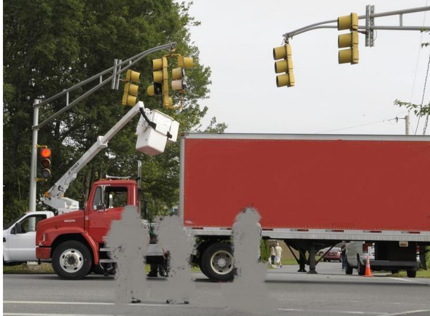
Figure 5 – Incident location after the incident showing the traffic signal, the aerial lift's raised buck and the semi-tractor trailer
