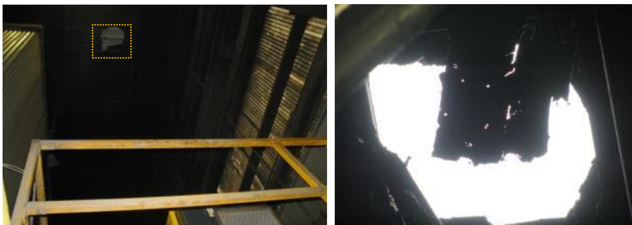
FIGURE 4. Pictures from inside plant, underneath where victim fell (left: hole had been repaired since the incident; right: close up of hole on day of incident).
