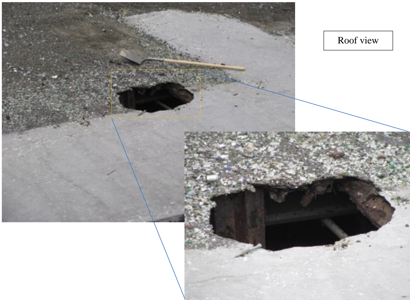
FIGURE 3. Close up of roof where victim fell.
