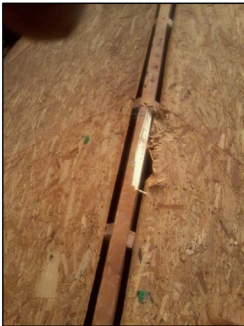
Photo 3. PFAS anchor location after incident ( Photo courtesy of NCDOL/OSH )
