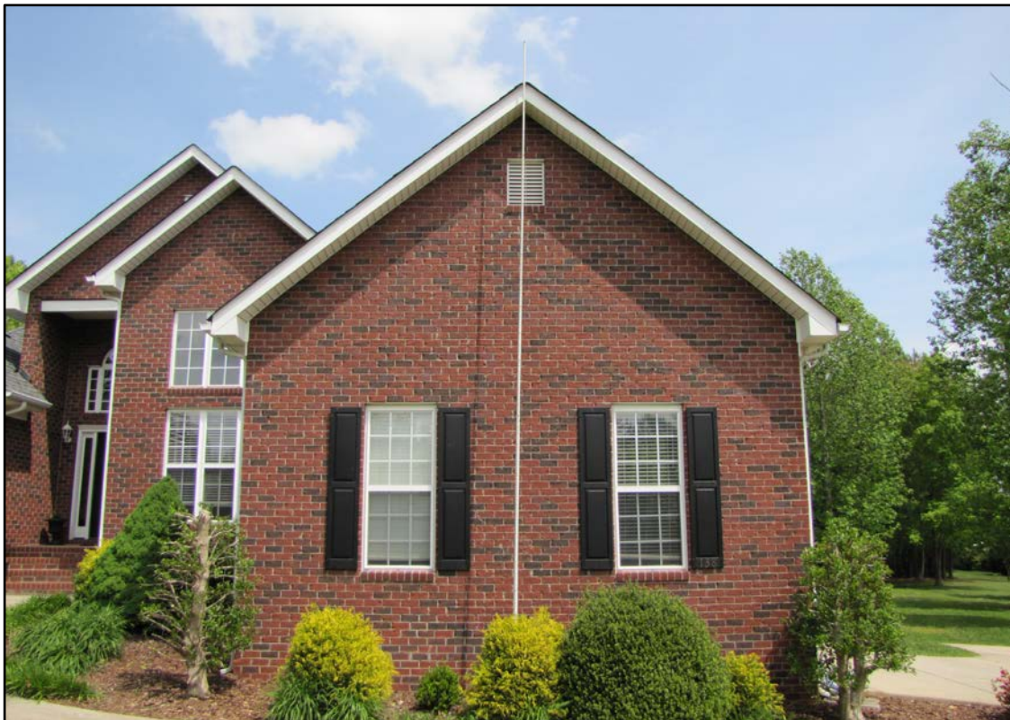
Photo 1. Roof pitch of the garage was determined to be 10/12 (Photo courtesy of NCDOL/OSH)
