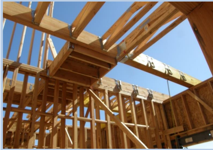
Photo of incident scene showing the opening the worker fell through while installing floor trusses.
