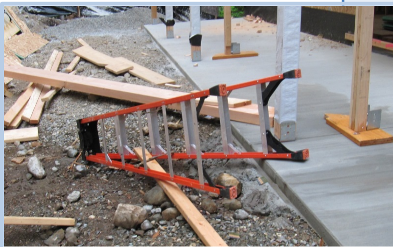
Incident scene showing the stepladder from which a carpenter fell and hit his head on the concrete patio. The ladder had been properly set up and placed on the patio.
