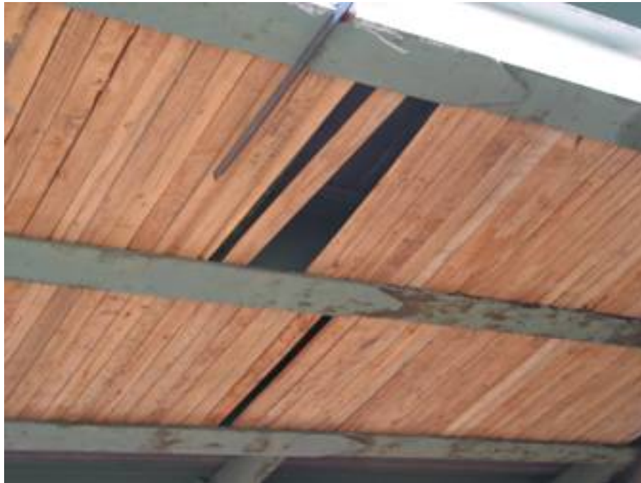
Figure 1. Example of shifting bridge deck “catch” platform wooden planks (view from ground).
