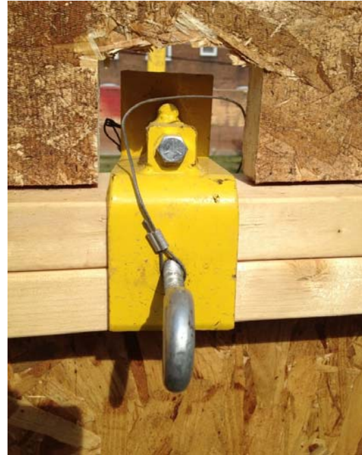
Figure 6 – Notching of wall scaffold bracket.
