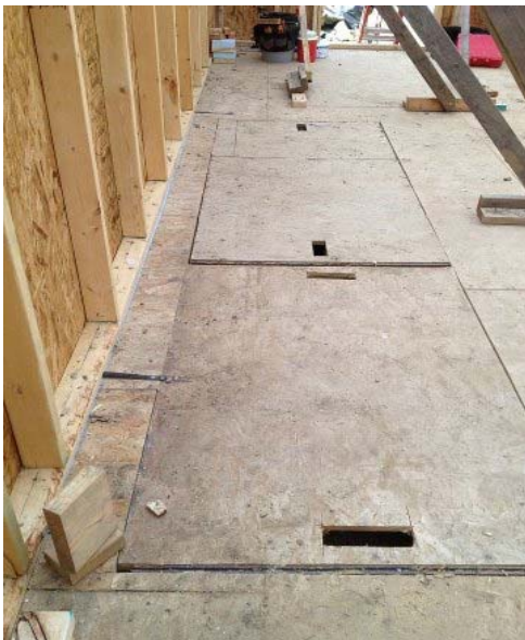
Figure 9 – Reusable sections of stair opening covers. Note: handle holes should be covered.
