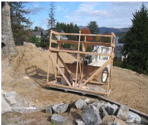
Photo 4 Two-tier Platform (courtesy of OSHA)
