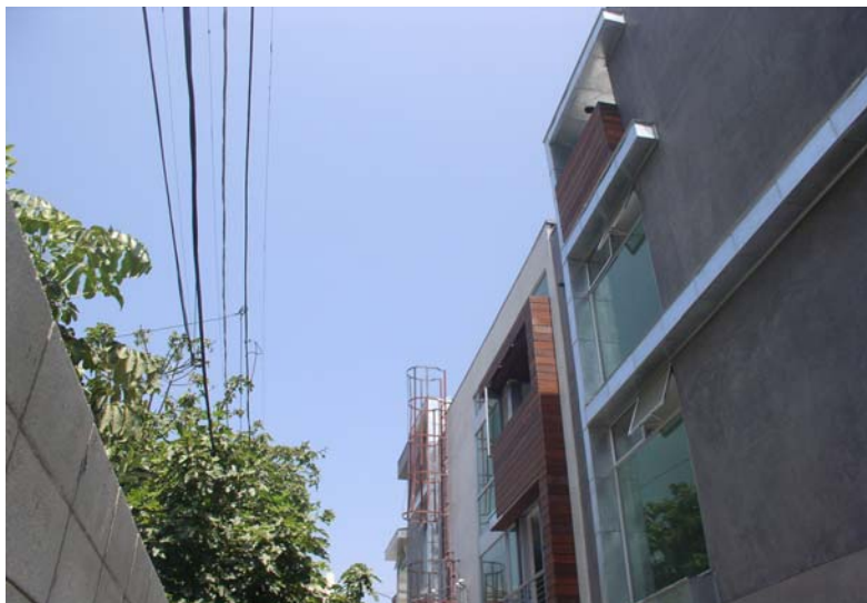
Exhibit 2. The top of the building under construction where the victim was working.
