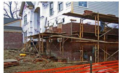
Example of poorly constructed scaffolding. Photo: courtesy of Robert Carr.
